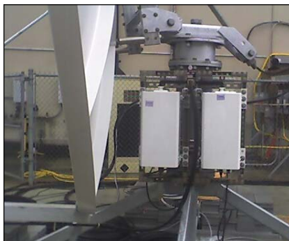
Antenna-mount 1:1 system w/ mounting frame
