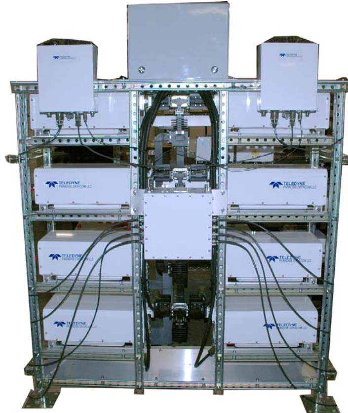
1.6 kW C-Band SSPA System configured with (8) 250W Modules
